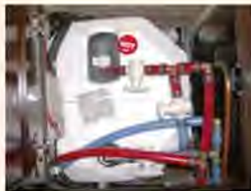
Summer Position / working water heater
